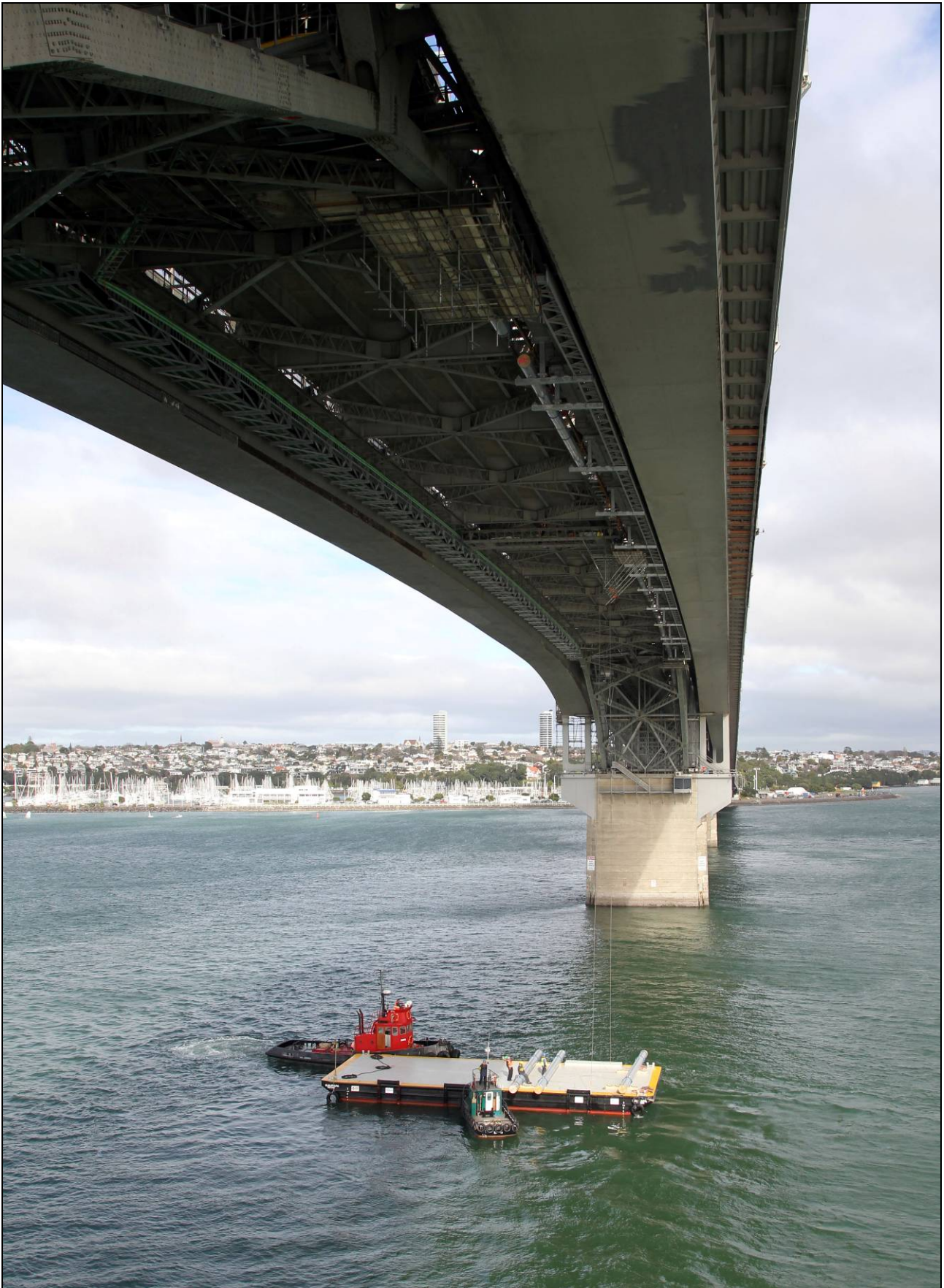
The North Shore No. 1 and No. 2 watermains, located under the carriageway of the Auckland Harbour Bridge, which supply drinking water to North Shore households and businesses, were recently lowered at the urgent request of the NZ Transport Agency to avoid the high risk of rupture due to the carriageway above flexing with traffic movement. The project required new pipes to be barged to the site and hoisted into position at the lower level so that the existing pipeline could continue to carry water to supply the North Shore.
